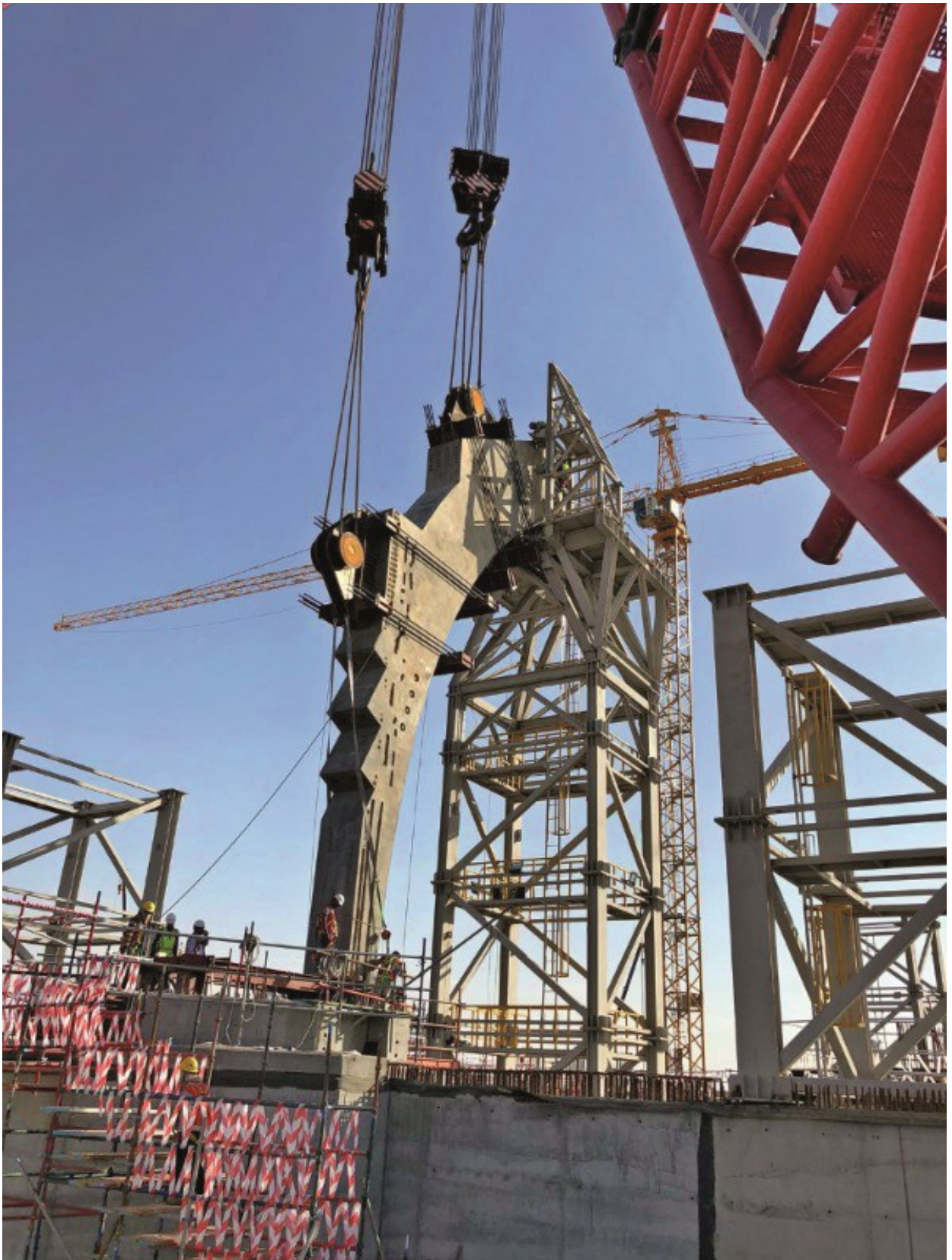
Mammoet is using nine crawler cranes for the construction of Kuwait International Airport
