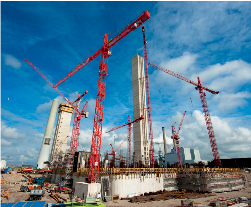
Wolffkran cranes, big and small, support the construction of a power station's core and walls in the Netherlands.
