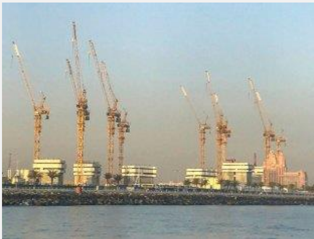
Manitowoc has 10 of its Potain MR418 machines being used for the first time in the UAE to construct the Royal Atlantis Resort and Residences
